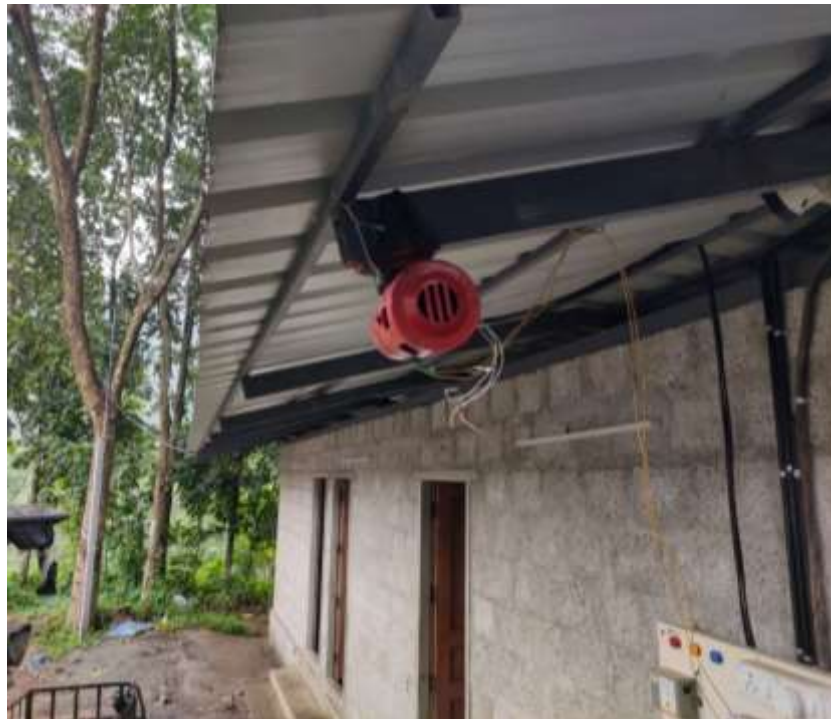
Figure 4: Photograph of Alarm
