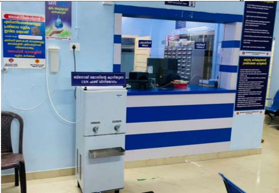
Figure 9: Photographs of Water Purifier Installed at PHC, Alakode
